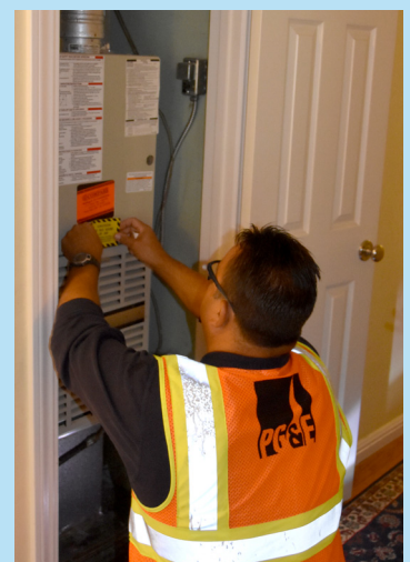
In Lafayette, gas service representative Doug Sutter provides a free gas safety inspection.
