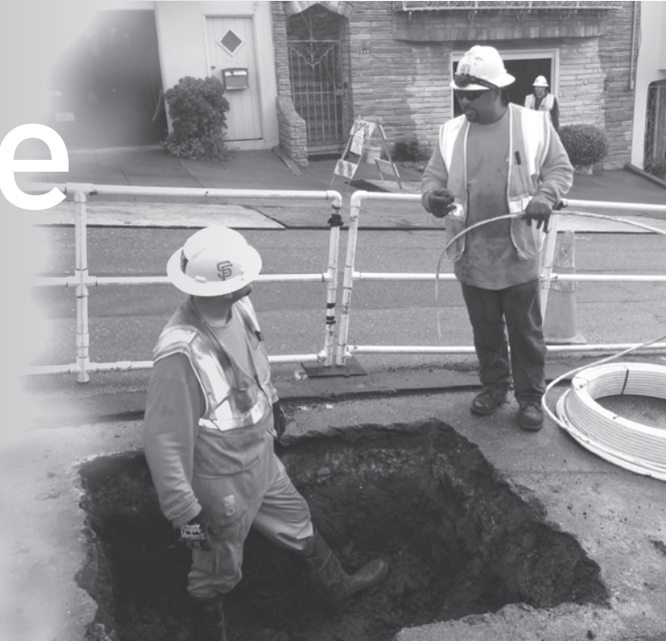
Replacing pipeline is part of PG&E's plan to upgrade our gas distribution system. Here, work on the system takes place in San Francisco earlier this year. (Photo by Nichol Carranza.)
