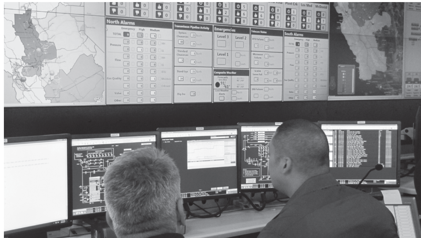
Gas-system operators have specific data on monitors at their workstations and a 90-foot video wall for situational awareness.
